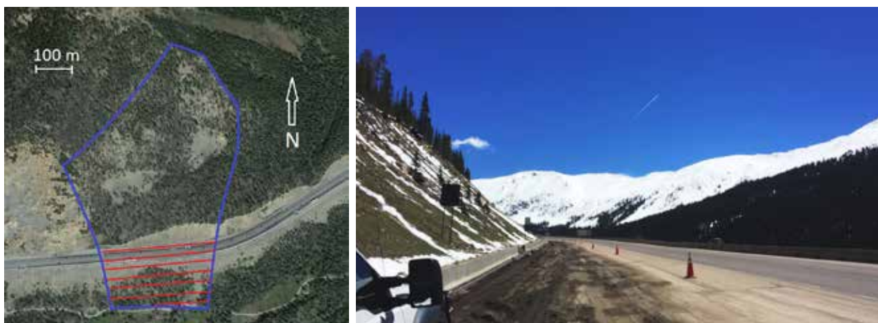
Figure 1. Aerial and ground-level photos of I-70 embankment fill. (Map data © 2018 Google Earth.)
