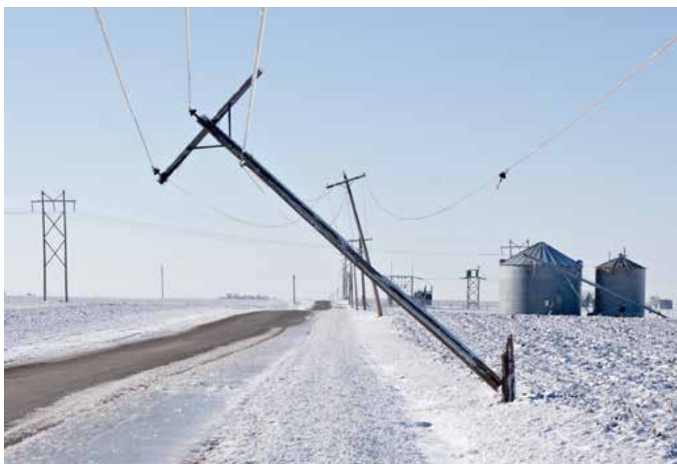
Figure 2. Broken power poles – moment capacity exceeded.
